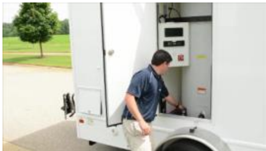
Pressure Gauge in Unit.
