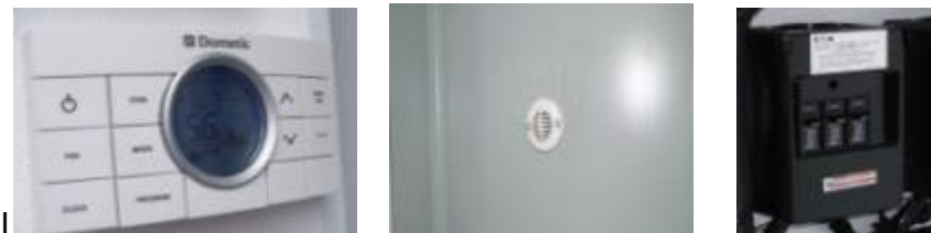
1. AC/Heat Control Panel 2. Thermostat Sensor 3. Men's and Women's Heater
