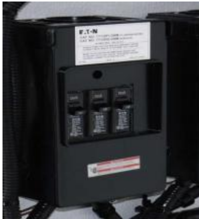
Turn on AC & Service Area Breakers
