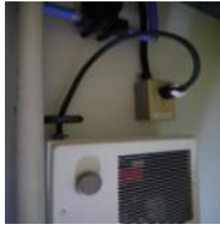
Service Area Heater
